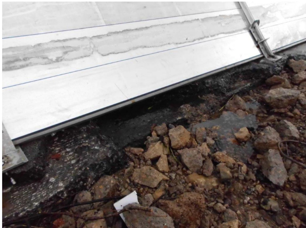
Figure 9: Photograph showing the exposed road edge and an area where the flood water has washed away tarmac and base material
