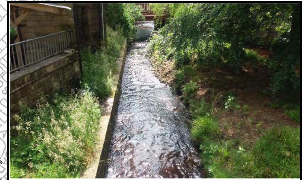
Walls around Innovation Mill will need to be raised and sealed, or property level provided
