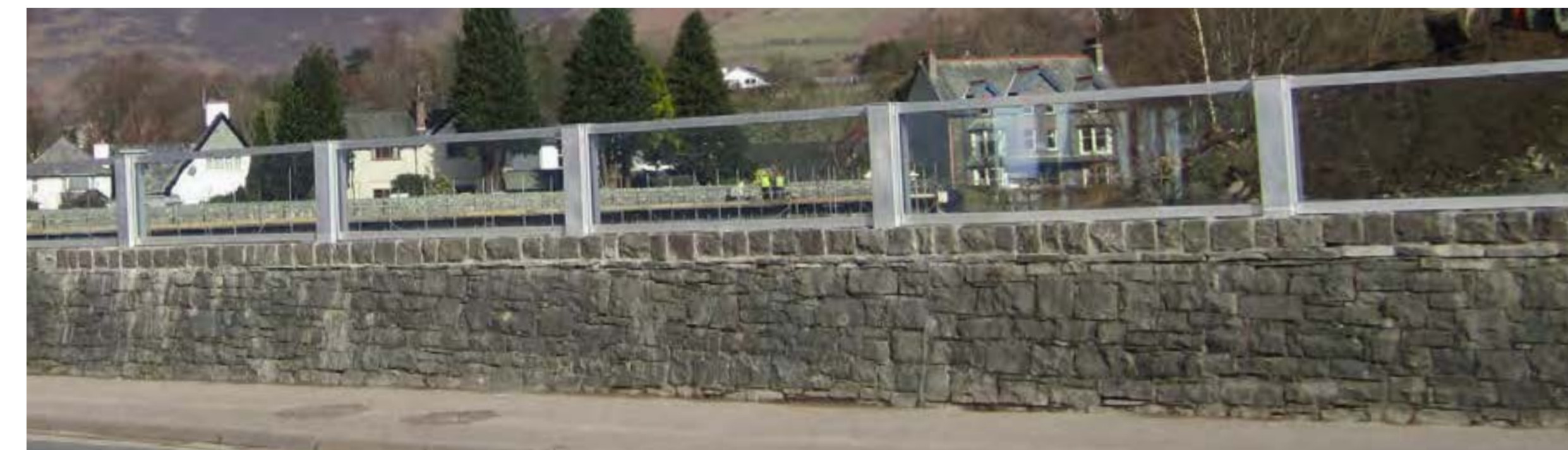
Stone clad flood wall topped with glass along its length © EA
