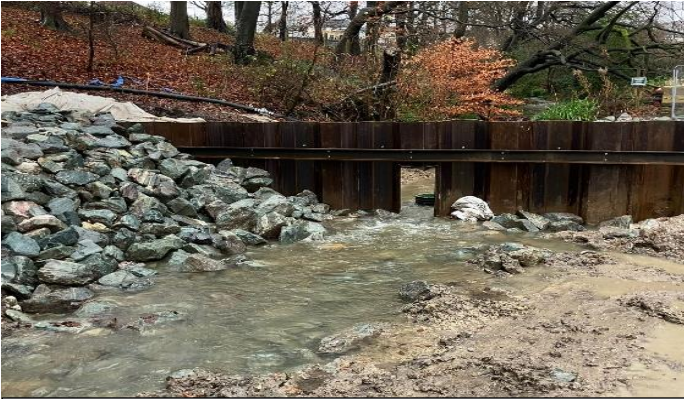
Flow control structure, with RIPRAP visible to the left side – Whinney Hill Park
